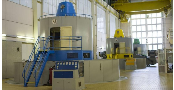
Figure 8 – Generators in the Orlik Hydroelectric Power Plant
