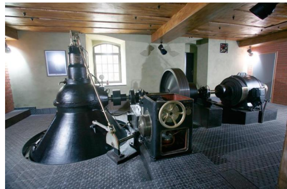
Figure 18 – Kalikovský mlýn Hydroelectric Power Plant
