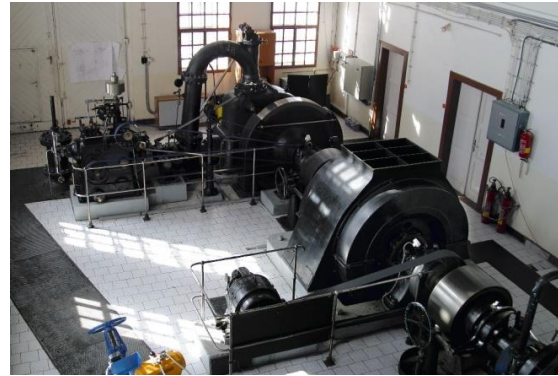
Figure 14 – Engine room of the Černé jezero Hydroelectric Power Plant
